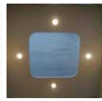
Skylight with LED Lights
