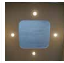
Skylight with LED Lights
